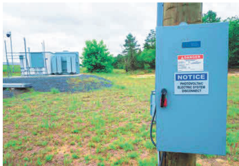
Figure 4-25: AC voltage measurements must be recorded at all connection points from the inverter output to the utility point of interconnection.
