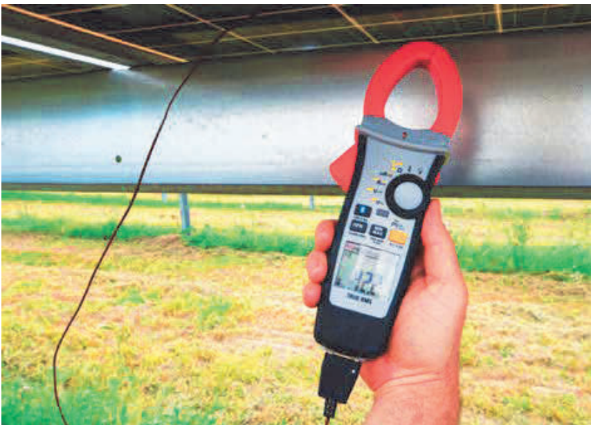
Figure 4-8: A technician measures the module temperature with a temperature sensor integrated into a DMM.
