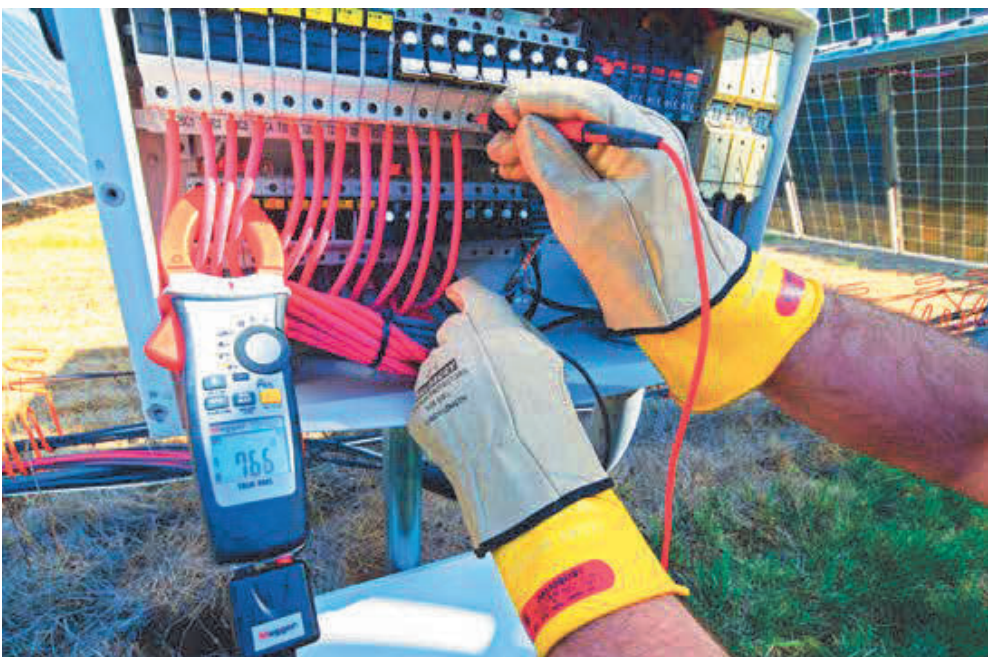
Figure 4-15: Technician recording voltage measurements at a PV array combiner box.
