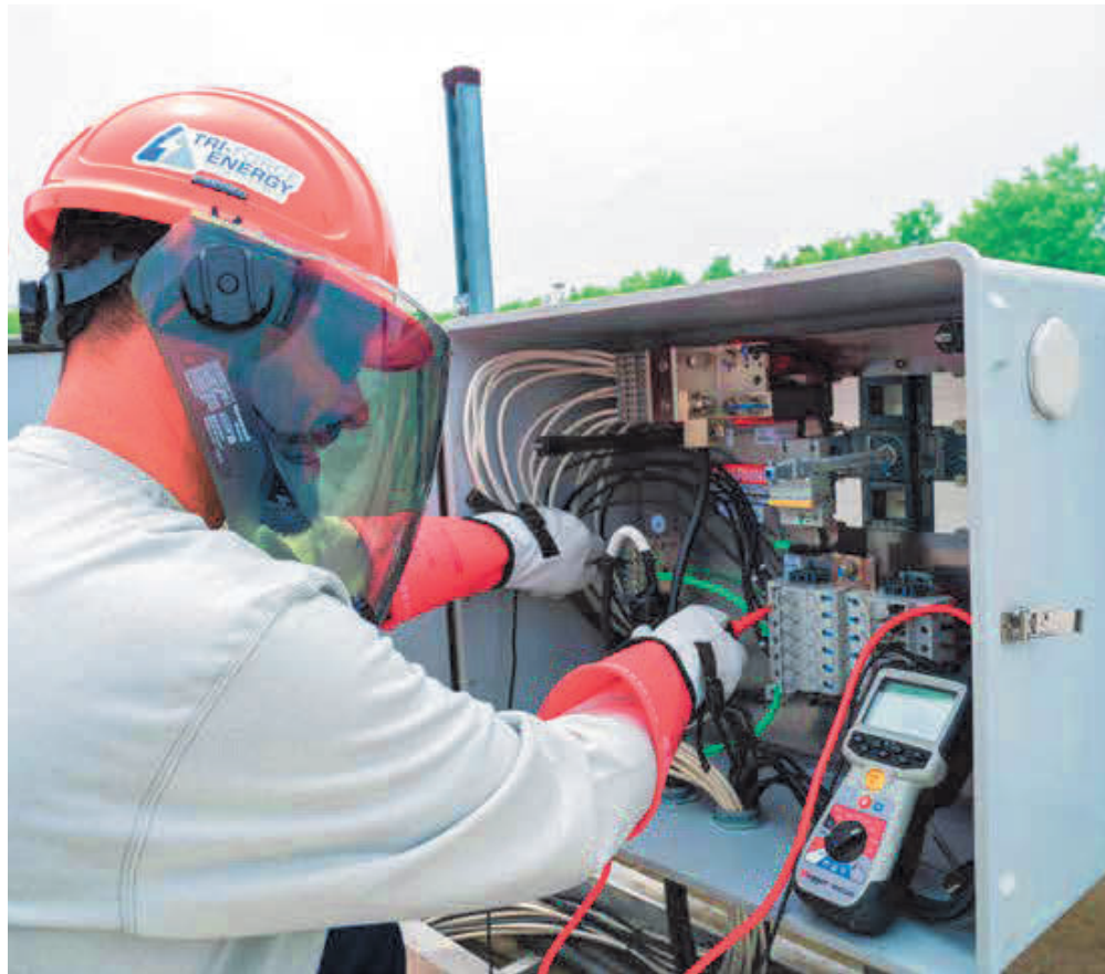
Figure 13-11: Technicians can estimate the point within a PV string where a ground fault has occurred by using the rated open-circuit voltage ( V_{oc} ) for the PV module and the voltage measured from positive to ground and negative to ground.
