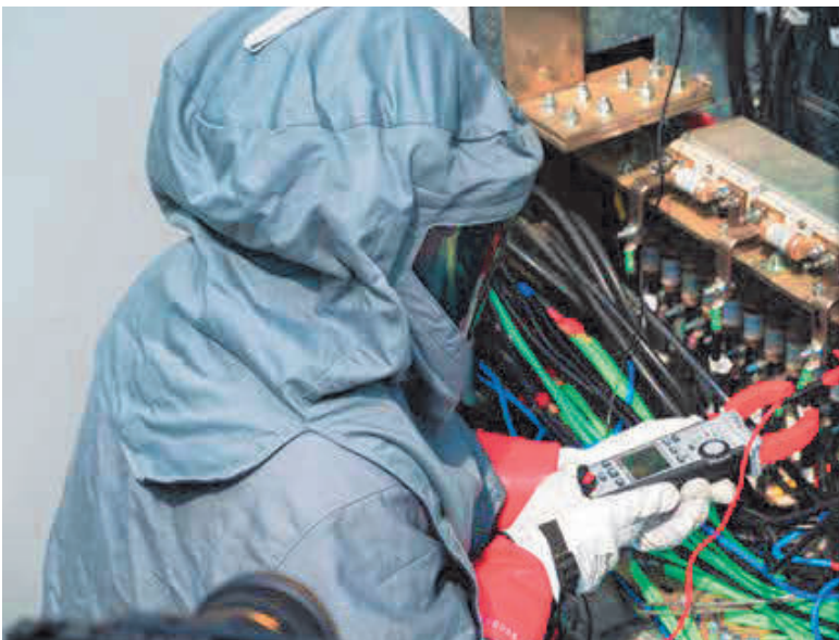
Figure 13-17: Verify no current is flowing on DC circuits prior to opening touch-safe fuse-holders.
