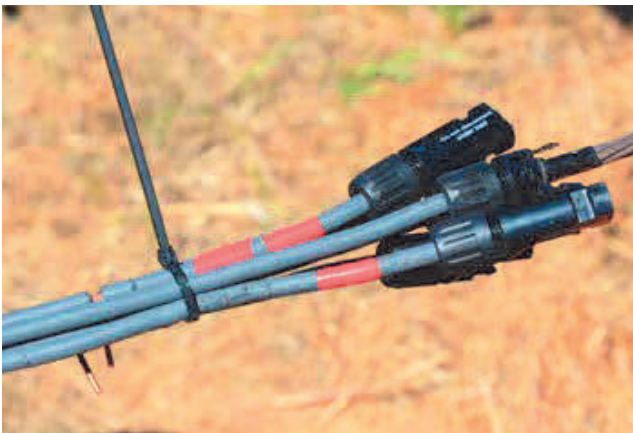
Figure 13-12: Once the fault location has been narrowed down to the string or combiner-box level, technicians should visually inspect the conductors in that region to look for signs of damage.
