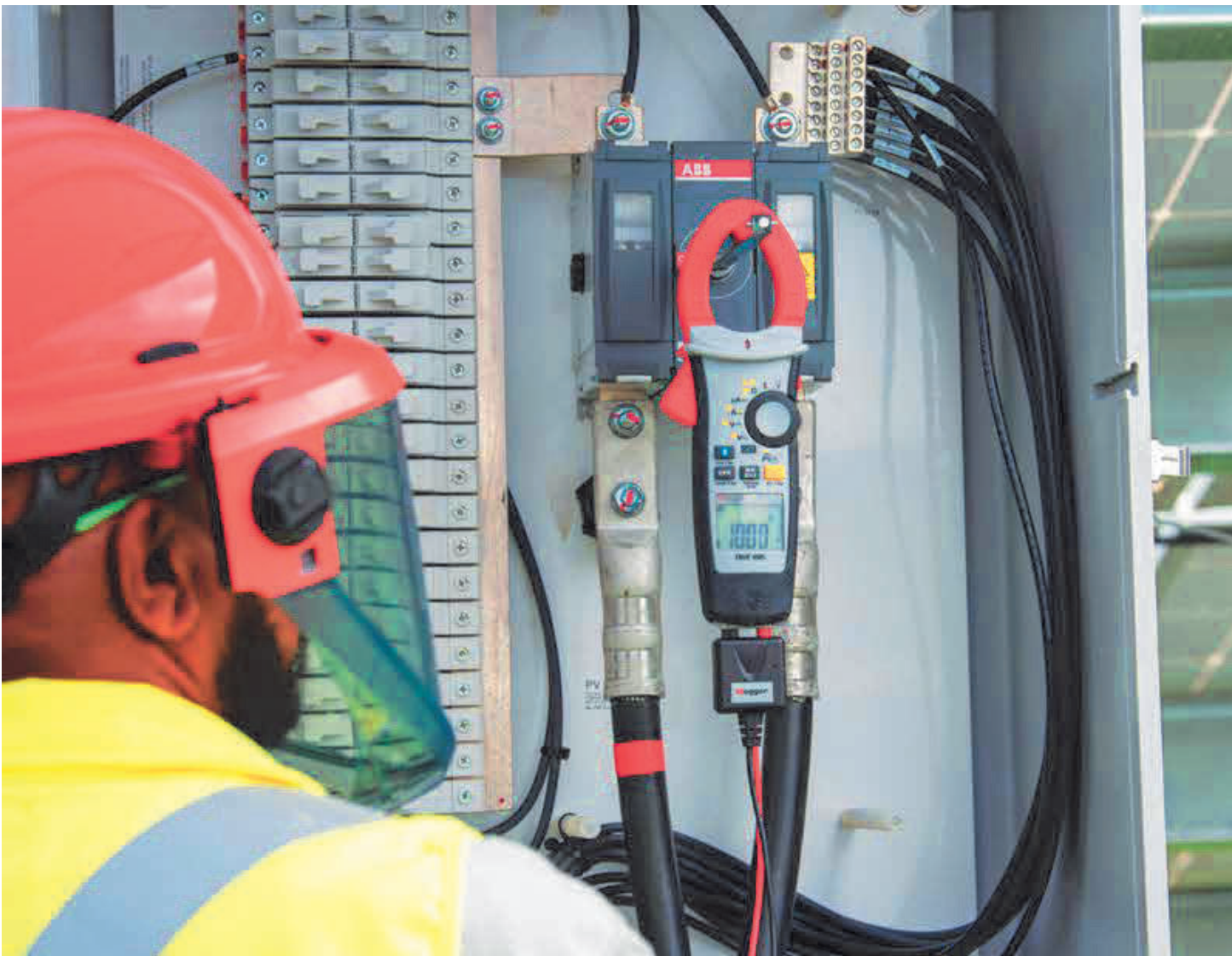
Figure 13-16: Technicians should proceed cautiously if a ground fault is detected onsite. At higher system voltages, fault currents increase, also increasing the shock hazard.
