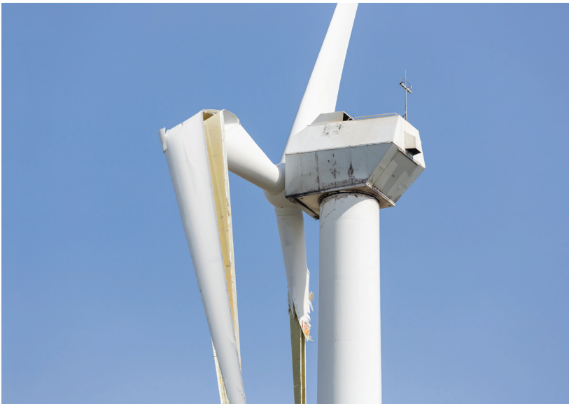
Figure 1a and Figure 1b: Lightning Damage to Wind Turbines
